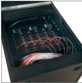
▲ Top Mount Patchbay with Littlite & Hot Pocket Circuit and Non-Dim Patch Panel
